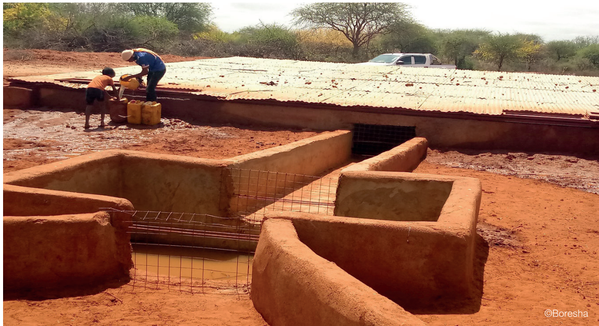
Figure 5: Underground storage facility, Mandera Kenya. PARS 2020
